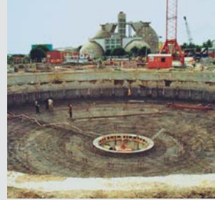
Industrial wastewater treatment plant
