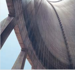
Natural draft cooling tower
