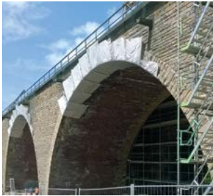
Renovation of the masonry at the Einsiedelstein bridge on the A1 motorway
